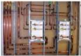
Medical Gas Pipeline
