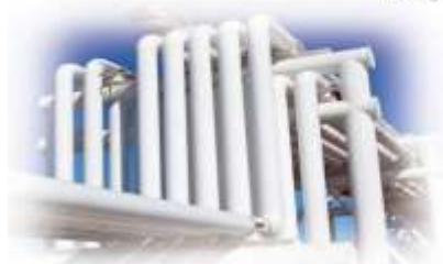
Industrial Gases Pipeline
